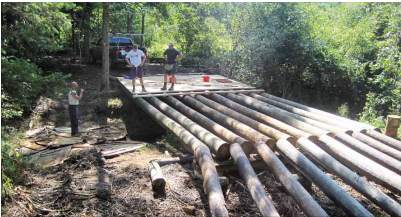
REEDS BROOK TRAIL SYSTEM NEARING COMPLETION —Hampden Academy senior Ryan Cole (center) and his father, David Cole, put decking on the bridge over Reeds Brook that Ryan has been building as his Eagle Scout project. The bridge is part of the Reeds Brook Trail System, which is under construction behind Reeds Brook Middle School. Thanks to a lot of volunteers, the trail system is almost complete. Hampden residents Kip Nelson (left) and Shawn Ramsay (not in photo) turned out for the first of two trail maintenance days on August 9. The second trail maintenance day is Saturday, Aug. 23. See story (reprinted from the July 31 Bangor Daily News) on p. 7.
